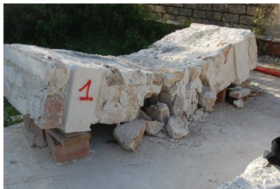
Figure 12. Failure of panel 1
